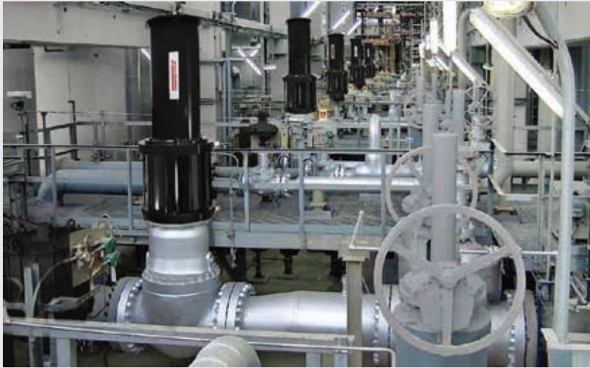
Fail-close AS Series on MP steam isolation valves in a HRSG at a US power plant
